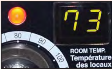
Temperature display and thermostat help control fuel usage
