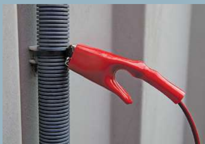
Small diameter cable tracing techniques
