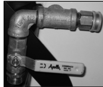
Figure 25: Left Water Valve
