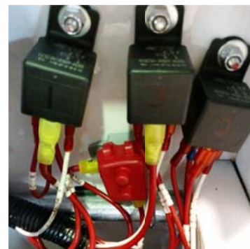
Figure 69: Circuit Breaker and Relays
