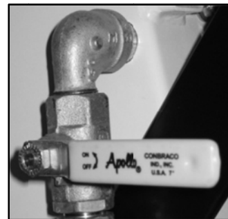
Figure 26: Right Water Valve
