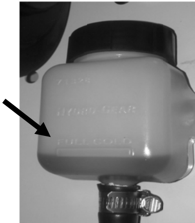
Figure 81 Expansion Tank Cold Line
