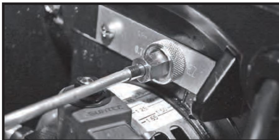
FIGURE 2B: OIL LINE FITTING
