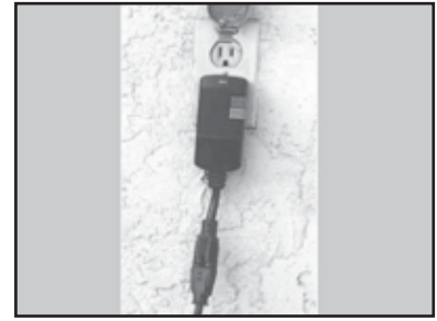
(C) Check Ground Fault Circuit Interrupter (GFCI) is not tripped
