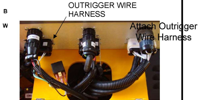
Figure 4-17. Bottom Side of the Ground (lower) Control Box.
