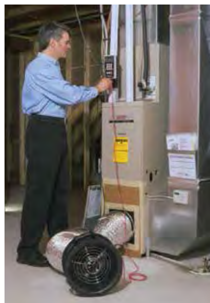
The Duct Blaster® can measure the total amount of air moving through the air handler.
