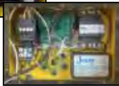
Electrical Junction Box
