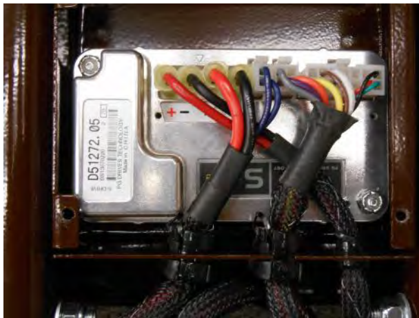
S-DRIVE BOX LOCATED ON CENTER OF CHASSIS
